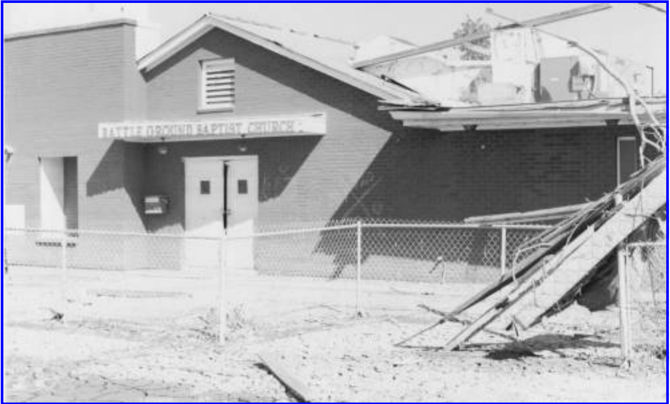
FIGURE 4. Battle Ground Baptist Church in the Lower Ninth Ward after Hurricane Katrina and the floods. The church is a brick shell because it has been thoroughly gutted. (J. Nash Porter, 2005).
