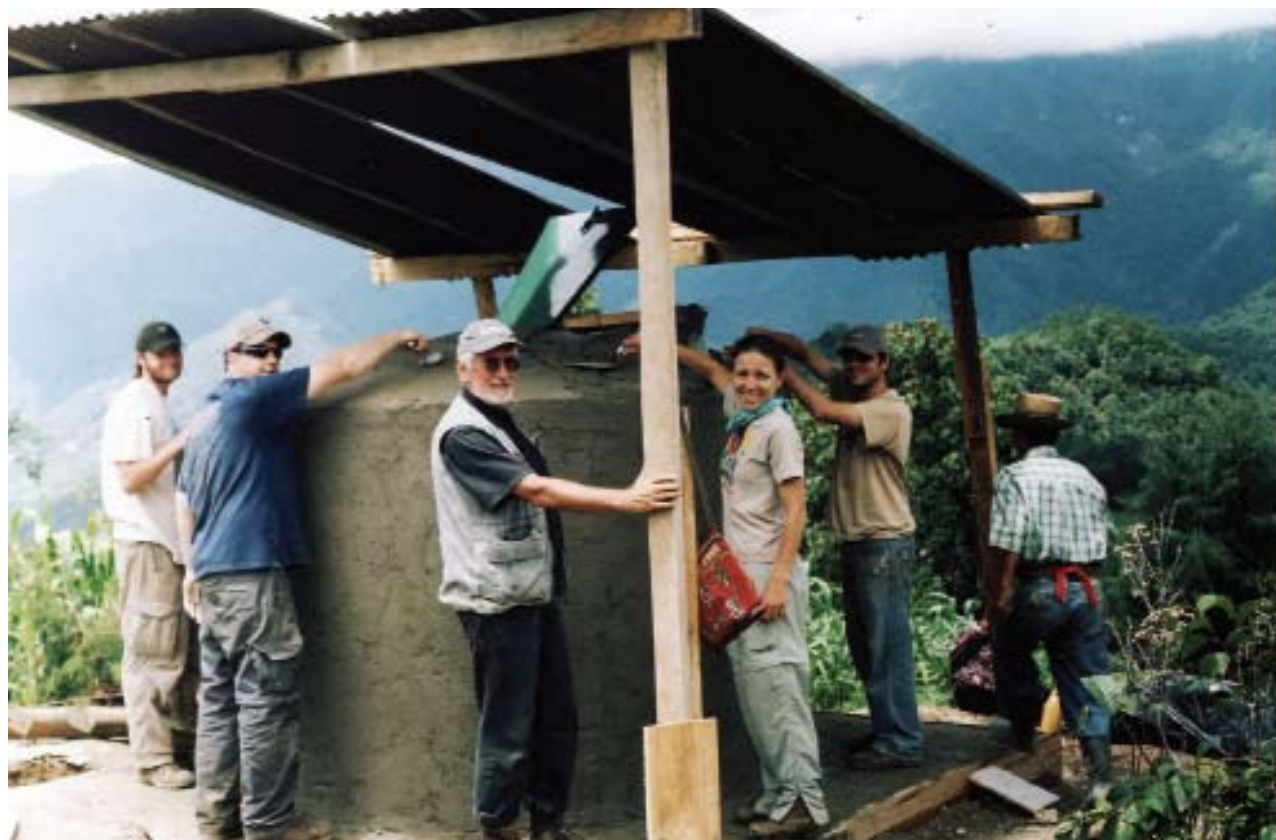
The pipeline built by students and residents of Quejchip connects springs on the other side of a mountain to this concrete distribution tank at the village's edge.
